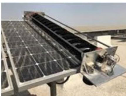
Figure 1. Solar photovoltaic station with self-cleaning and foiling system.
