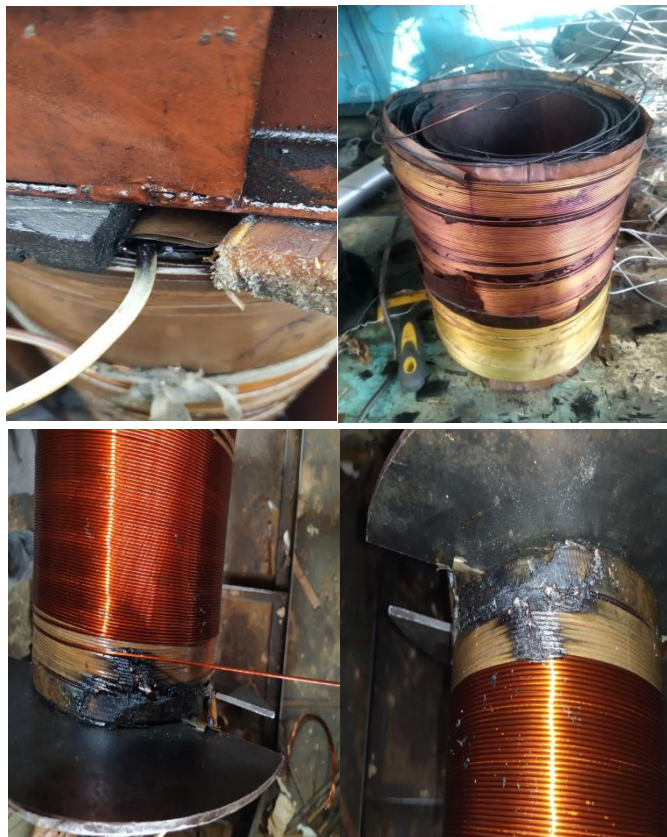
Figure 1. Burned and damaged cases of the transformer core.
