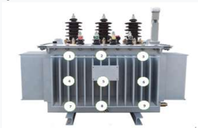
Figure 1. Points for measuring the level of vibration of the wall of the transformer tank.
